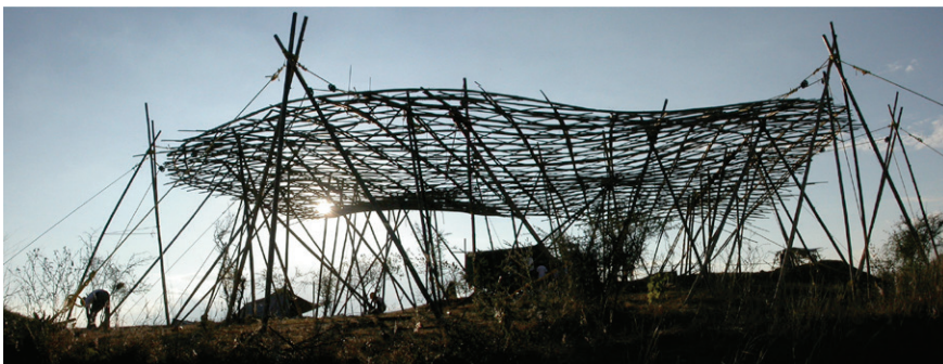
Techo en México, Studio Prix – Special Projects ; University of Applied Arts Vienna The bamboo roof is held in shape by scaffolding, poles, and rope / Feb 2004, Oaxaca, Mexico
